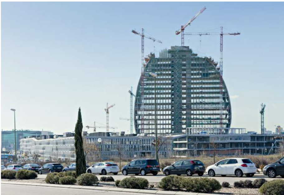
The high-rise accentuates the visibility of BBVA to the outside world. Its soft contours and transparency make it appear fragile and delicate
