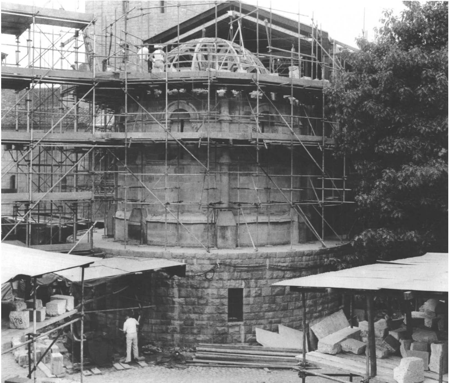
46 The apse during reconstruction at The Cloisters with the centerings in place. In the foreground are racks containing the numbered stones
