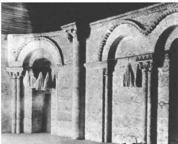
38 The upper part of the south wall of the choir of the church of Notre-Dame-du-Bourg at Langon being used for the drying of tobacco (1934)
