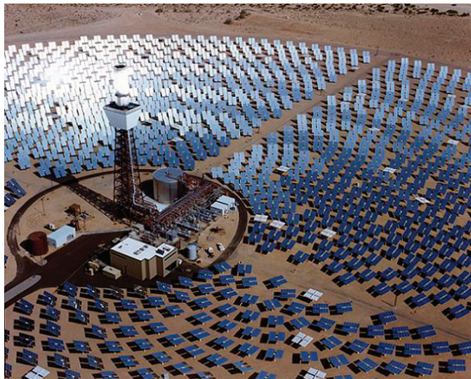
FIGURE 5.2.1 In this photograph of a concentrating solar power (CSP) technology, stretched membrane heliostats with silvered polymer reflectors will be used as demonstration units at the Solar Two central receiver. The Solar Two project will refurbish this 10-megawatt central receiver power tower, known as Solar One. SOURCE: Image available at https://www.eere.multimedia.energy.gov/solar/ .
